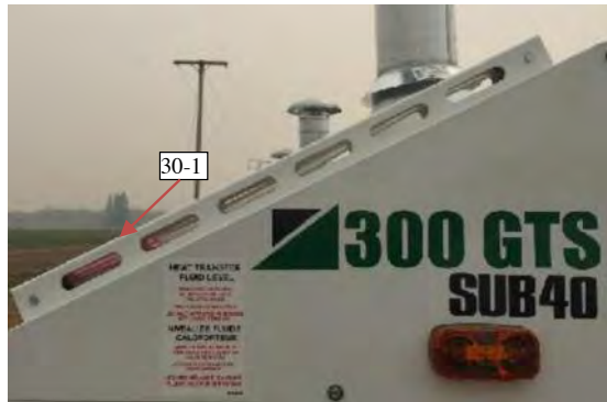
31-Glycol level sight gauge
