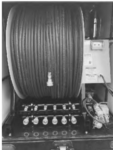
2 - TD300 Central Mobile Enclosure (back view)
