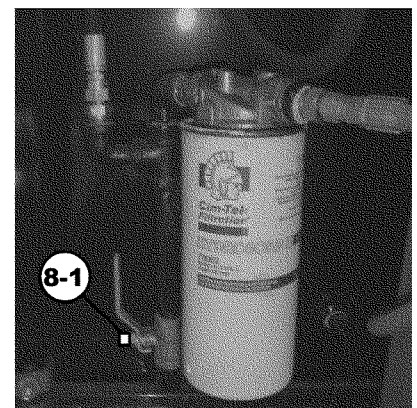
8 - fuel supply valve and filter
